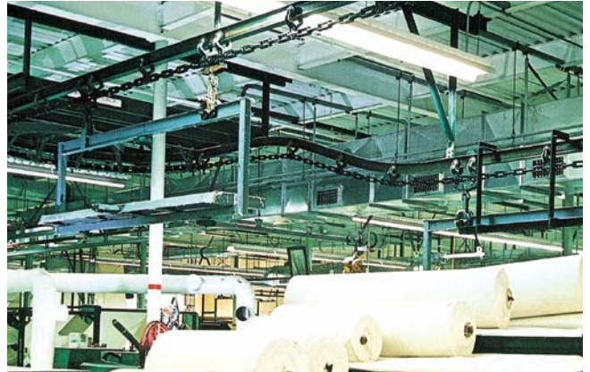
Trolley conveyor system
