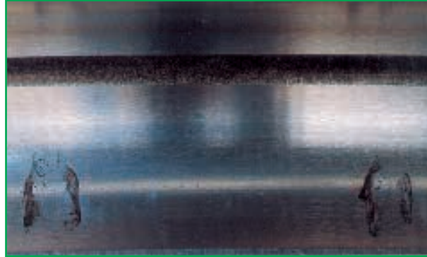
Fig. 6 Part: outer ring of a slewing ring Symptom: rust on raceway surface at ball pitch Cause: moisture condensation during stationary periods
