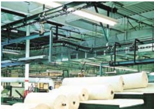
Trolley conveyor system
