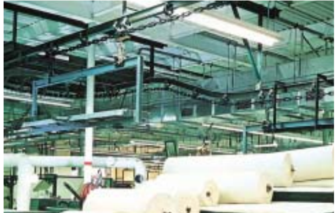
Trolley conveyor system
