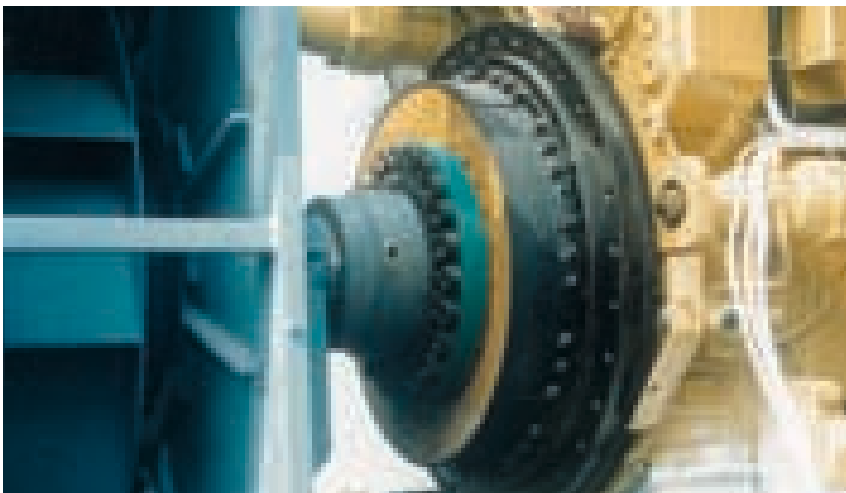
CX-80-BFS1 on genset an Generator
