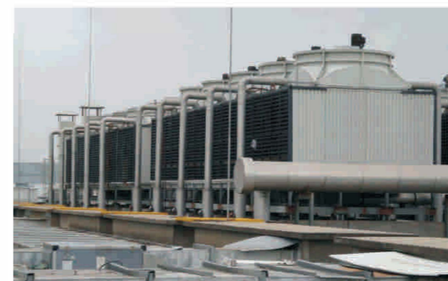
Hvac and water supply
